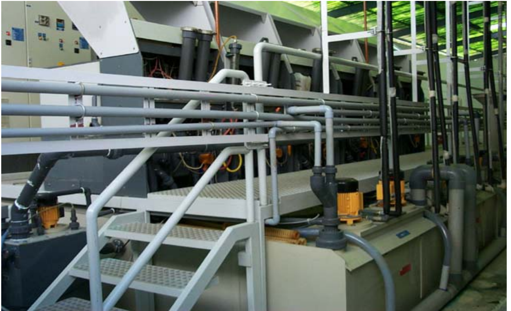
Set-up of process and storage tanks under the cells
