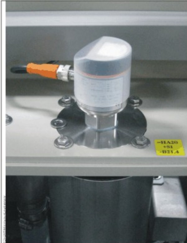
Microwave level sensor mounted on top of the module with help of a flange plate
