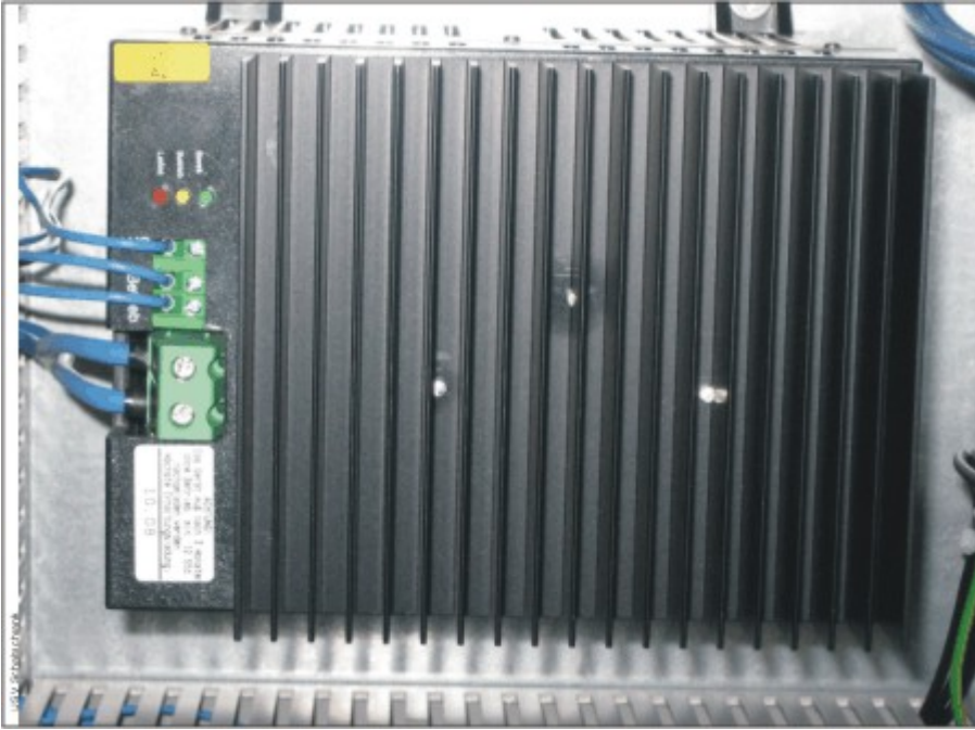
UPS unit in the control cabinet
