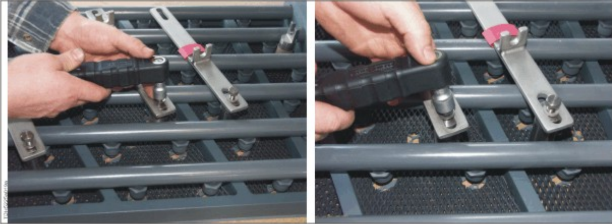
Fixing the color-marked connection bars to distance bolts with a defined torque
