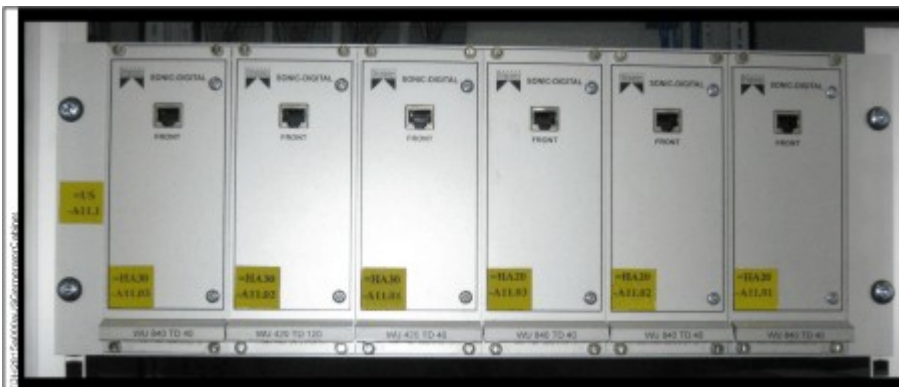
US-generators as aligned in the switch cabinet
