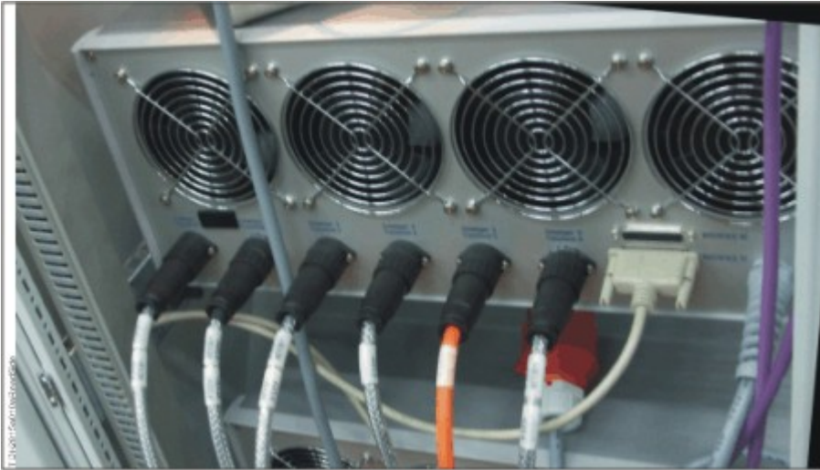
Transducer connectors on rear side of US-generator rack
