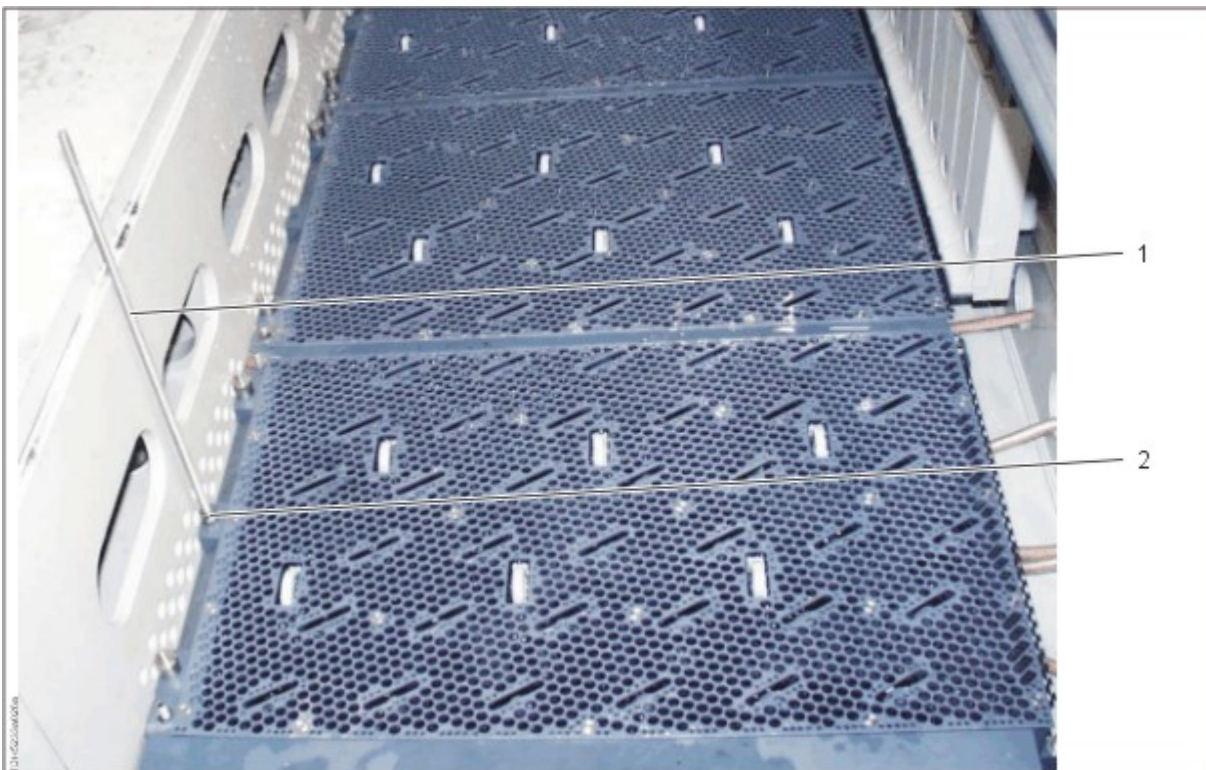
Auxiliary rod screwed in a threaded hole at the window side of the anode unit
