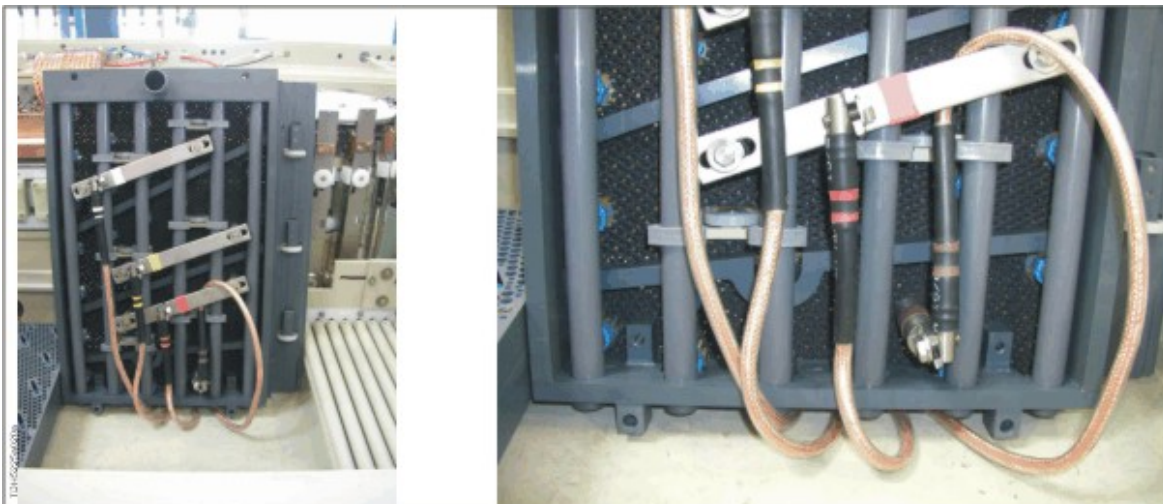
Bottom anode unit lifted for disconnection (later on reconnection) of the electric supply cables
